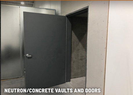
NEUTRON/CONCRETE VAULTS AND DOORS
